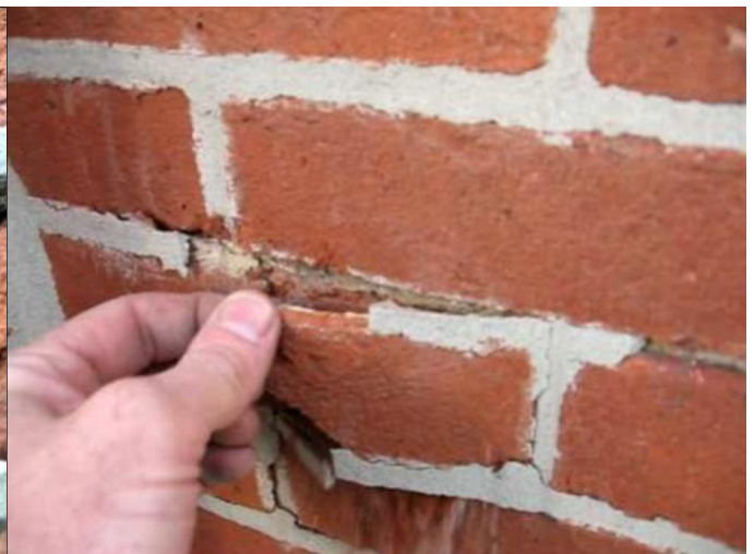
Above- Spalling brick, surface falling off
