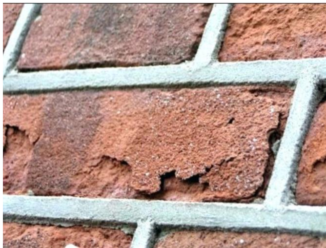
Above- Bricks are deteriorated, note mortar is still intact, bricks likely not the correct type for this application
